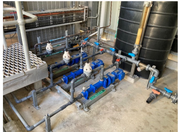
Figure 14: A cationic-polymer dosing system is used as a coagulant to improve the efficiency of clarification and separation processes.
